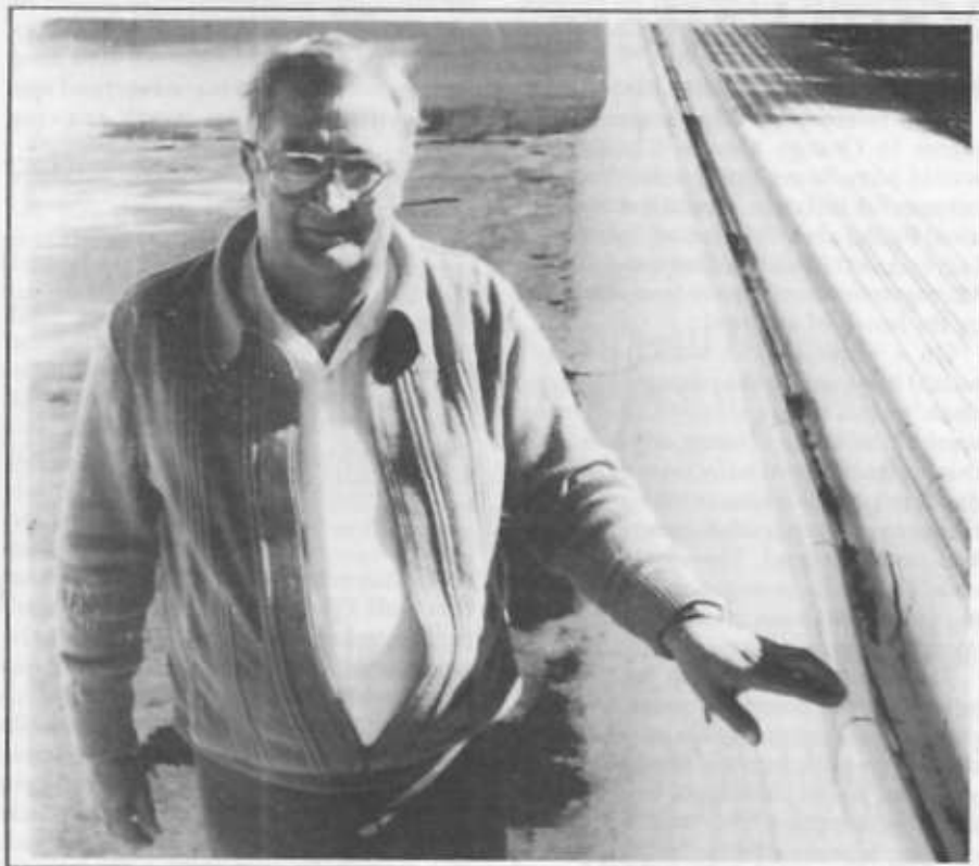
Ron Whiteley, standing in the town pool in the shade of the trees that have caused the damage, indicates the cracks.
