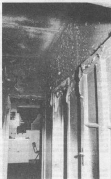
Blistered paintwork and charred walls in the hallway show the tremendous heat generated by the fire.
