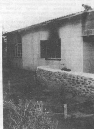
Fire blackened walls of the 4th Avenue house.
