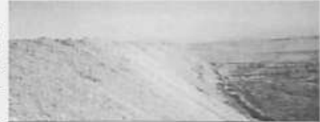
A PARALLEL VIEW OF THE SEAWALL AT G70 SHOWING THE MINI MINE (EAST OF THE SEAWALL)
