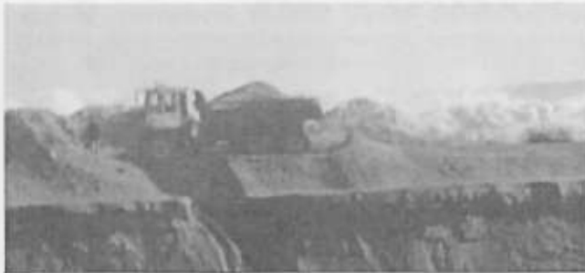
TOUGH TIMES! THE ROUGH SEA BASHING AND ERODING THE SEA WALL AT U105 WHICH CAUSED FLOODING OF THE MINE.
