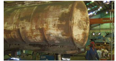
TANK IN THE WORKSHOP
