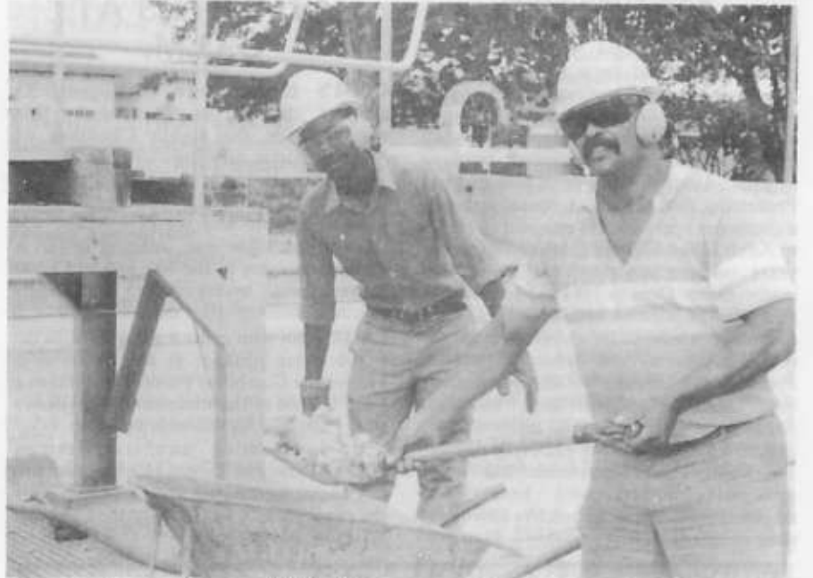
Contractors Johannes August and Willem Links tearing up the paving surrounding the town pool.
